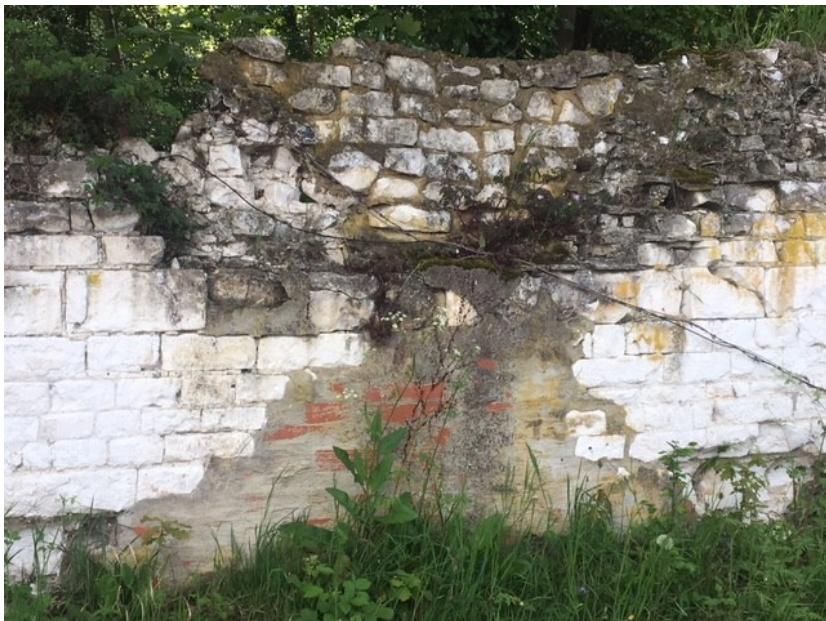
The Durdans Stables Clunch Wall – Previous repair work unsatisfactory
